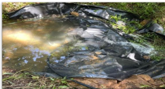
Overflow of water on constructed dam
